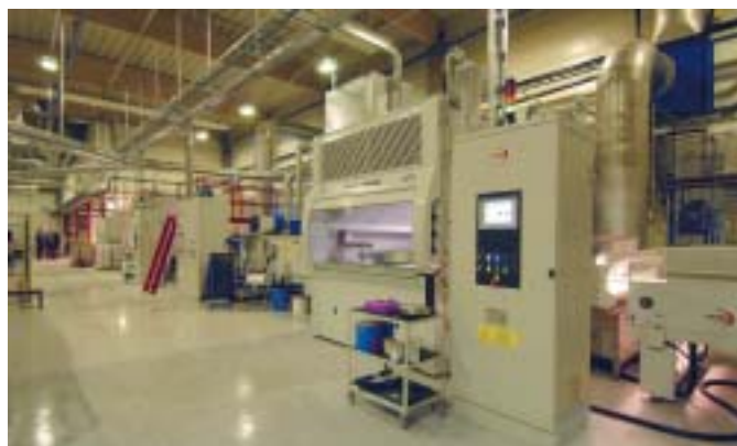
New surface treatment production line at Moelven Eidsvoll AS.
